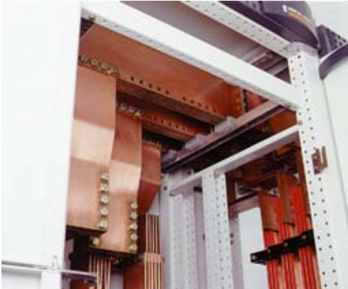
3200A 母线 3200A busbars
